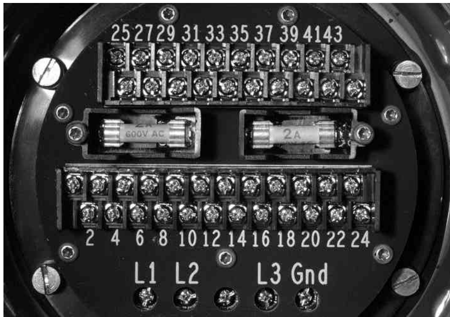
Figure 7-1 Fuses in the STC
