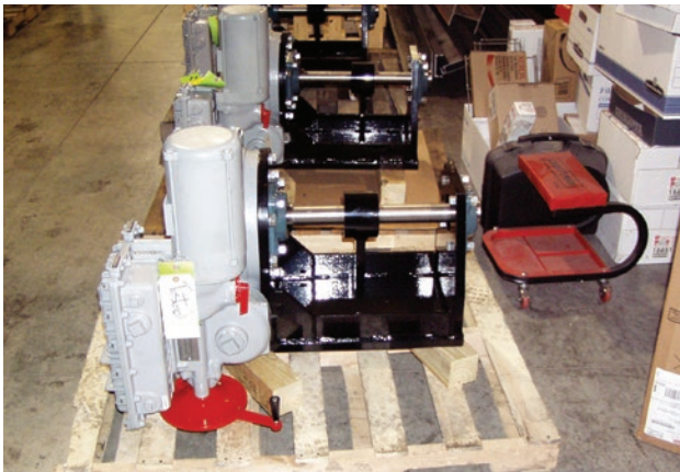
Bunker room, 3-position coal diverter gate drive
