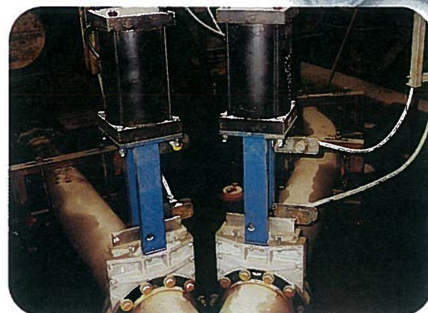
VALVES FOR ASH TRANSPORT LINES
