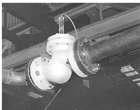
Figure 8 Size 4 Class 600 90° bonnet piston lift check valve with two upstream elbows (out of plane). This arrangement produces swirl as shown in Figure 7.
