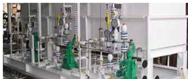
Chemical Injection Skid
