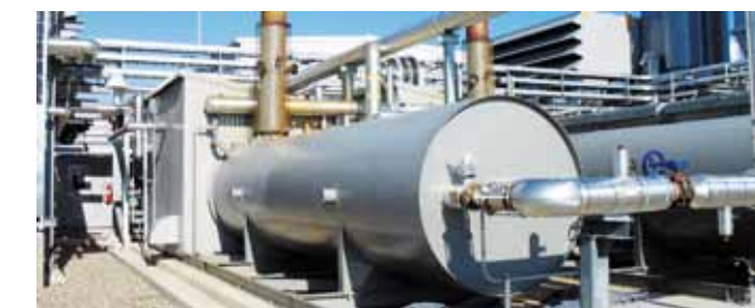
Indirect Water Bath Heater
